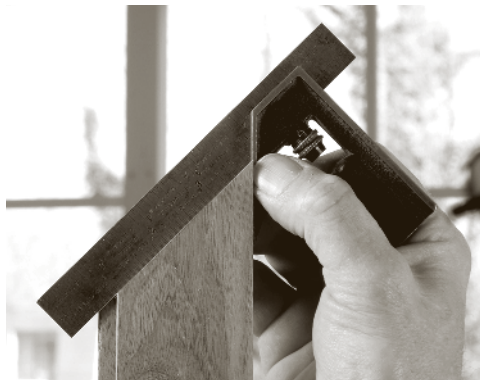
An accurate cut is essential. Check with a good square, holding the angled piece up to a source of light.
