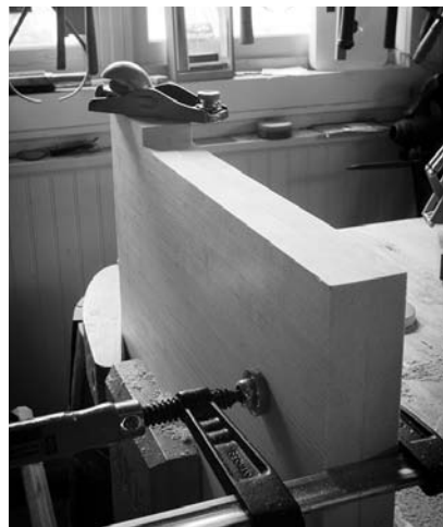
A plane job. Most of the clean-up of the notches is with a plane. Work to your layout lines and then clean up any excess in the corner.
