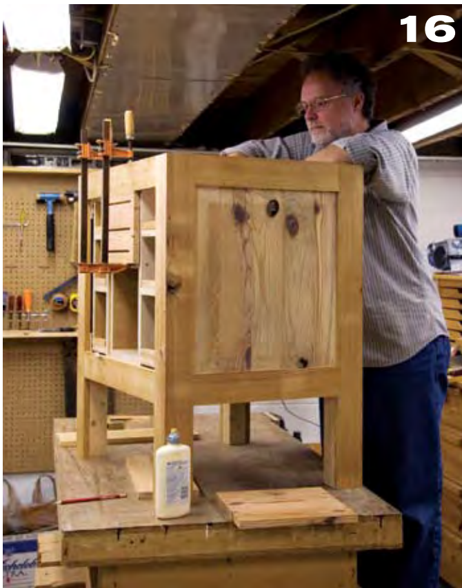
Glued the vent panel to the bottom of the top rail. Drill oversized holes in the side cleat and install one screw through each of the cleats. The panel is free to move with the seasons because the screws will move in the oversized holes.
