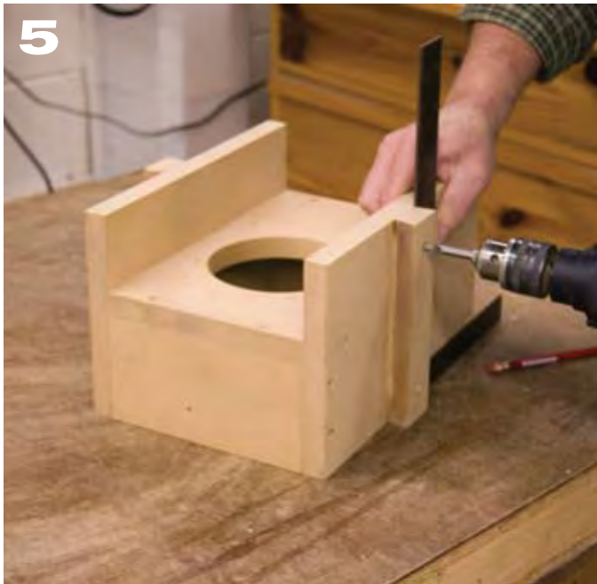
5 In the deck plate, center and cut a hole that is \frac{1}{2} " larger in diameter than your router's body. Assemble the box. Then attach the dovetailed guides, centering them on the inner side parts. Make sure they are square to the inner sides.
